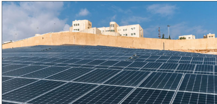
Light for light The solar plant powering SESAME, the synchrotron light source in Allan, Jordan. Since 2019, SESAME has been the first accelerator in the world to run entirely on renewable energy.
