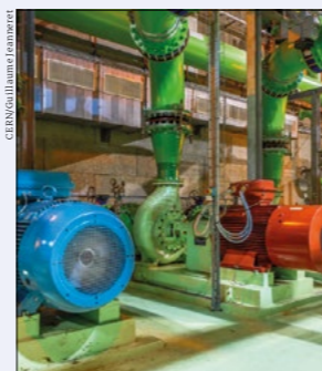
Stay cool An innovation partnership with industry aims to reduce the energy footprint of CERN's cooling and ventilation infrastructure. Above: cooling equipment used for the ATLAS experiment and the Super Proton Synchrotron (SPS) accelerator.
